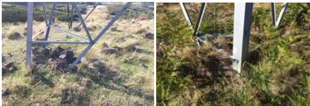
Figure 5.4 : Extensive footing backfill carried out in areas of displacing soils (Kalaga and Yenumula, 2016)
