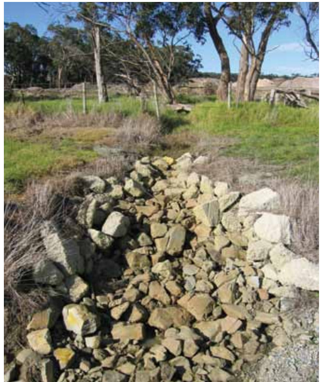
Rock lined discharge point to prevent erosion.
